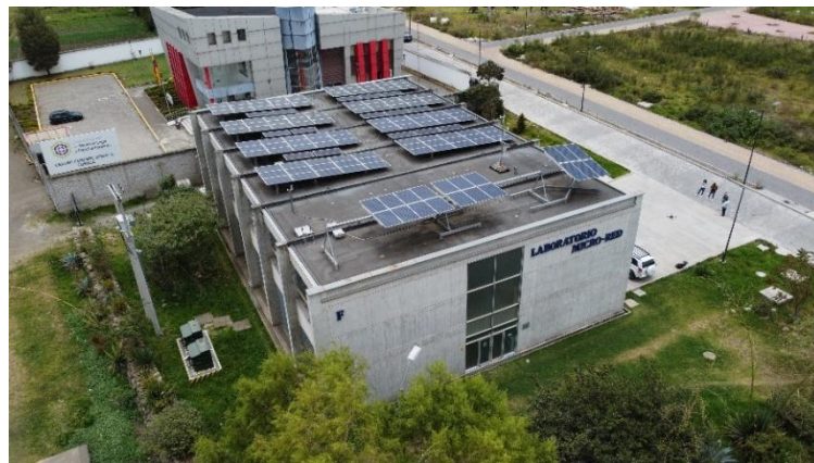
Figure 2. Rooftop PV installation (35 kWp) connected to the internal distribution panel.
